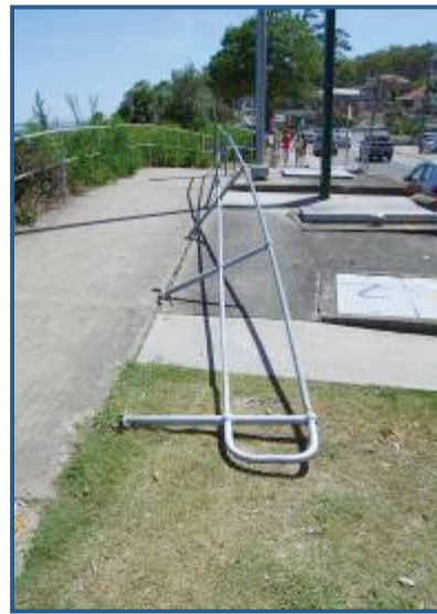
Damaged rail along sewerage station
