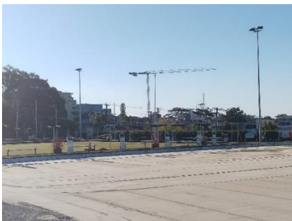
View of site (crane) from Nelson Bay Bowling Club entry level (Sept 2021)
